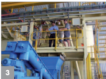
3 The final concrete mix is combined from two differently coloured mixes, using exact proportions according to colour specifications of the product
